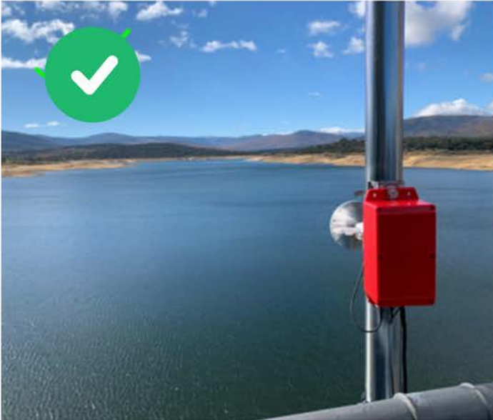
Good Installation: Clear field of view to the water with no obstruction.
